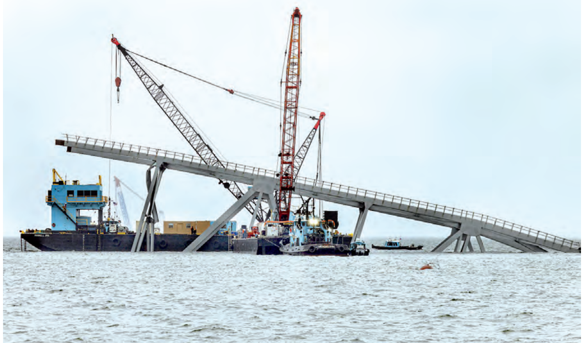
Cranes continue salvage work as wreckage of the Francis Scott Key Bridge rests on the container ship Dali, Wednesday, April 3 2024, in Baltimore.
