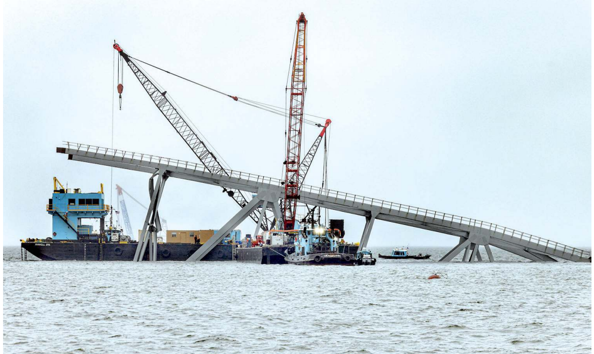
Cranes continue salvage work as wreckage of the Francis Scott Key Bridge rests on the container ship Dali, Wednesday, April 3 2024, in Baltimore.
