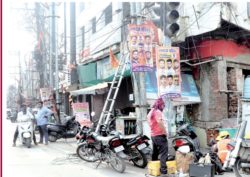
The linemen of the electricity department have started clearing the bunch of electrical wires from different chowks and localities to make it underground.
