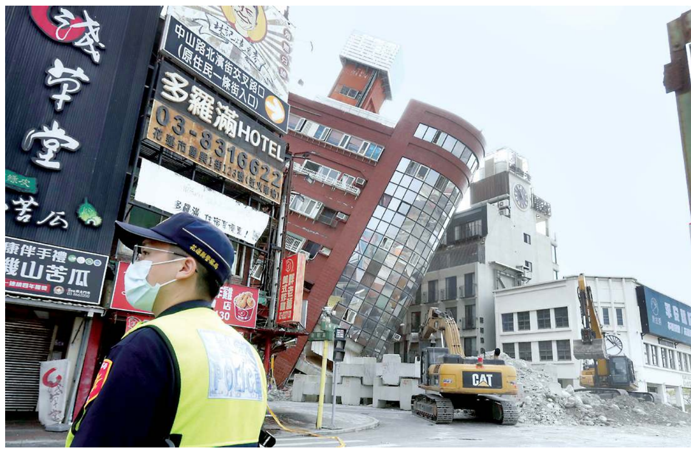
A police officer stands guard near a partially collapsed building a day after a powerful earthquake struck in Hualien City, eastern Taiwan, Thursday, April 4.
