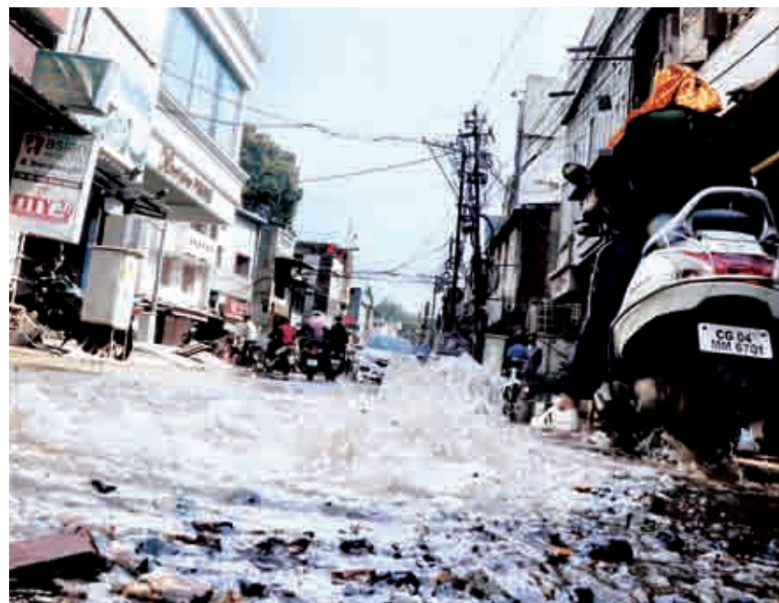
With bursting of water pipeline in Chotapara led to waste of gallons of drinking water in the middle of road here on Thursday.
