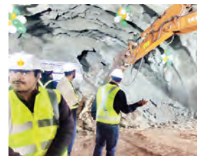
Engineers and workers during breakthrough ceremony of Naushera tunnel project, in Jammu & Kashmir, Sunday.
