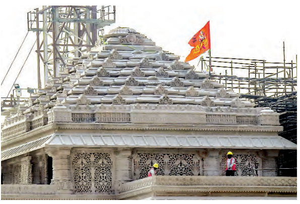
Under-construction Shri Ram Janmabhoomi temple during a media tour organised by Shri Ram Janmabhoomi Teerth Kshetra, in Ayodhya, Tuesday.
