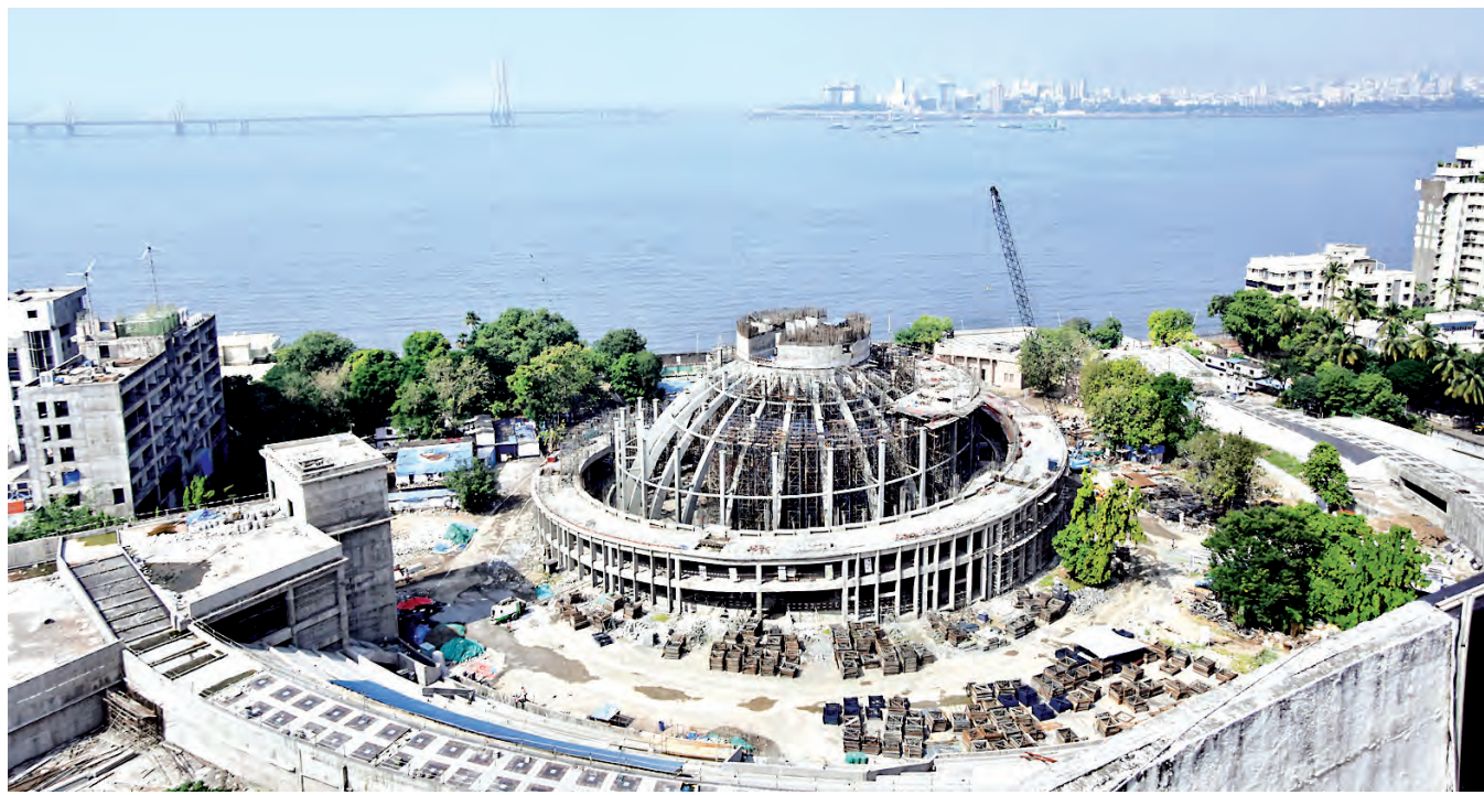
A memorial to B.R. Ambedkar being constructed at Dadar, in Mumbai, Thursday, Nov. 30.
