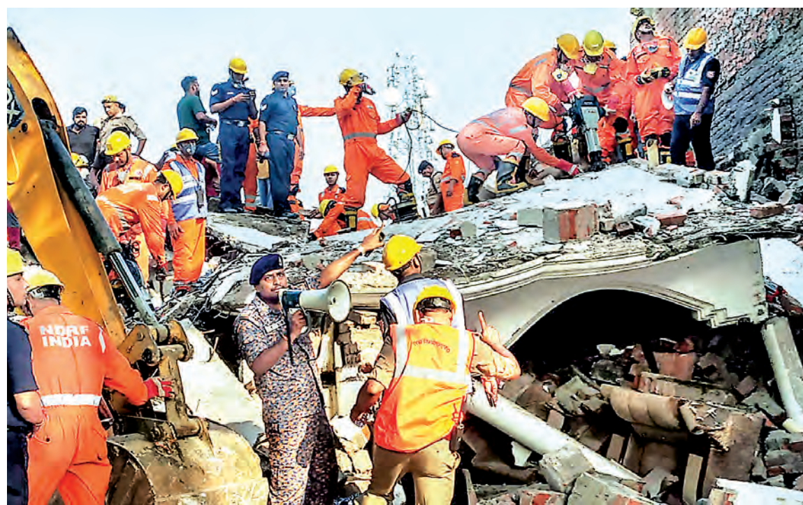
Rescue operation underway after a three-storey building in the Fatehpur area collapsed, in Barabanki district, Monday, Sept. 4.
