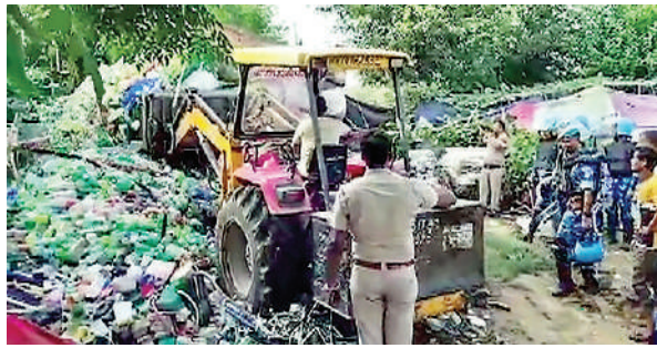
Police use heavy machinery to demolish shanties in Tauru near violence-hit Nuh.
