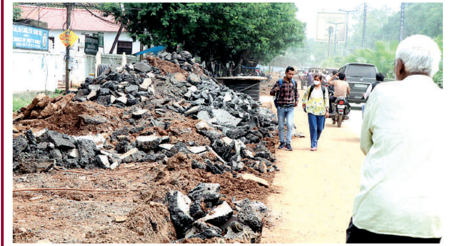
The debris after digging of road for laying of cables and pipeline has been left by the road-side by RMC without about the inconvenience being caused to the citizens
