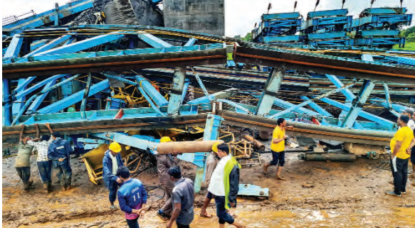
Police, locals and other Emergency Services personnel at the site after a girder launcher collapsed during the construction of a viaduct for the Samruddhi Expressway, in Thane district, Tuesday.
