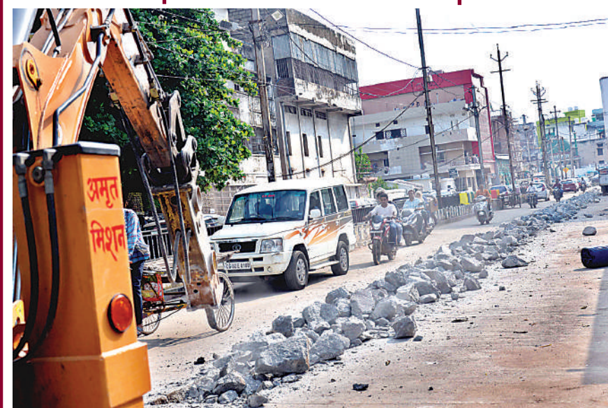
The digging of roads during peak of rainy season continues by RMC authorities for laying of water pipelines in different localities.
