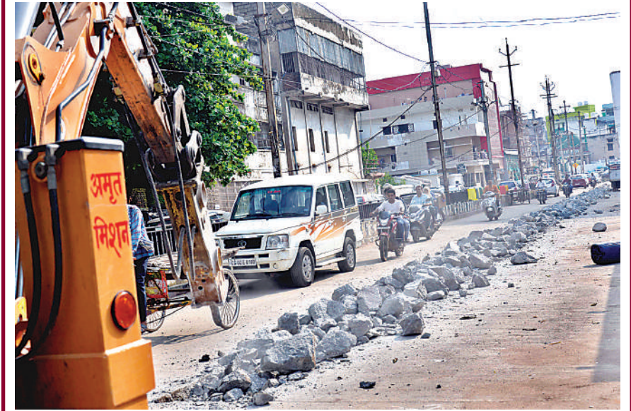
The digging of roads during peak of rainy season continues by RMC authorities for laying of water pipelines in different localities.
