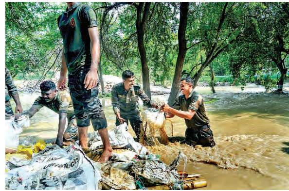
Army personnel carry out repair work after the drain regulator at ITO damaged due to flooding in the area by the Yamuna river, in New Delhi, Friday.
