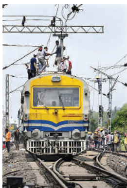
Restoration work underway at the site of the accident involving three trains, near Bahanaga Bazar railway station in Balasore district, Sunday.
