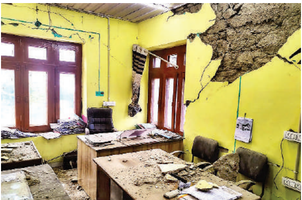
Damage at an office a day after a massive earthquake struck Chenab region, in Doda, Wednesday.
