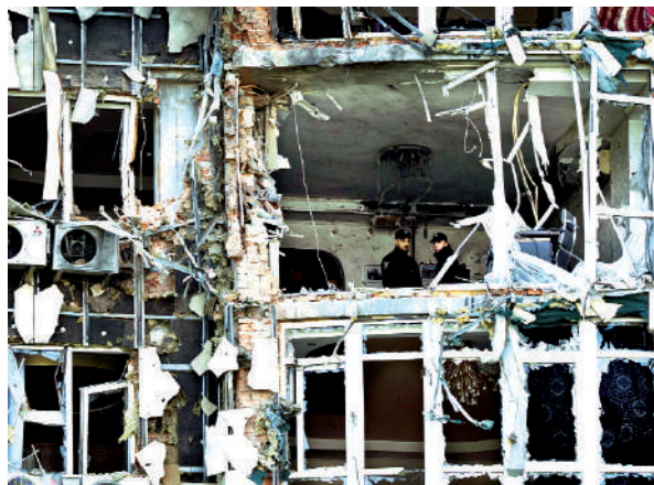
Police inspect an apartment building damaged by a drone, that was shot down during a Russian overnight strike, in Kyiv, Ukraine, Monday.
