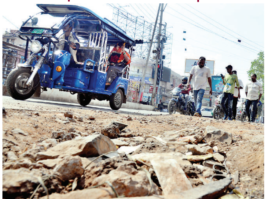
The digging for laying of pipeline and other has left the road uneven and posing threat to some accident during slipping of tyres.
