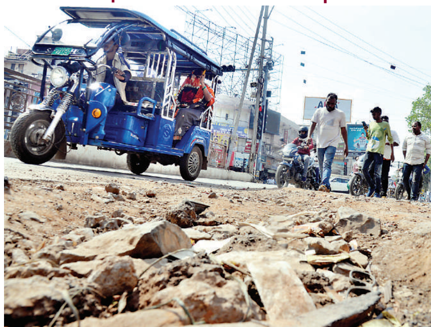
The digging for laying of pipeline and other has left the road uneven and posing threat to some accident during slipping of tyres.
