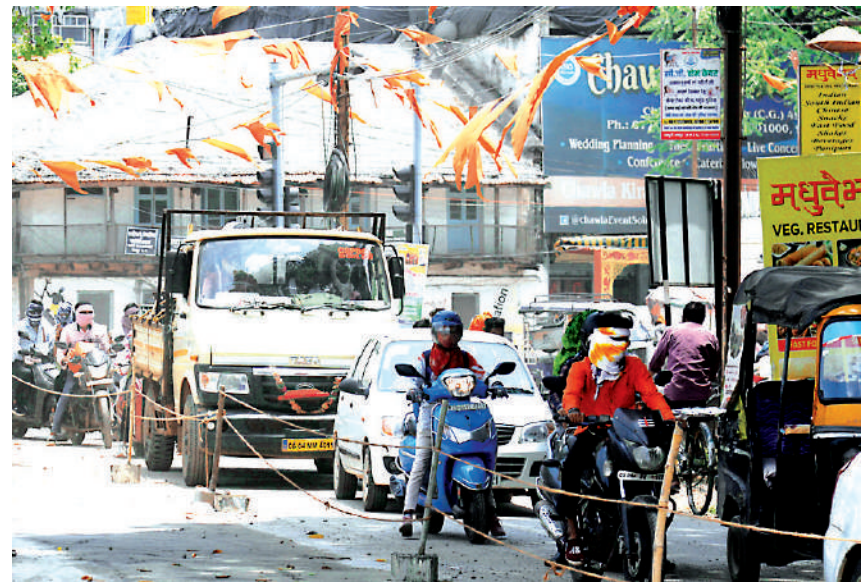
With digging work for laying of pipelines and others going on every nook and corner of city, people are made to face lots of inconvenience at Fire-brigade chowk, near Motibagh here on Thursday.
