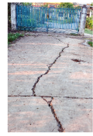
Path in village Kareli Badi is also in a similar condition, with most of the CC roads built during the former Sarpanch period being dilapidated and breaking down.
