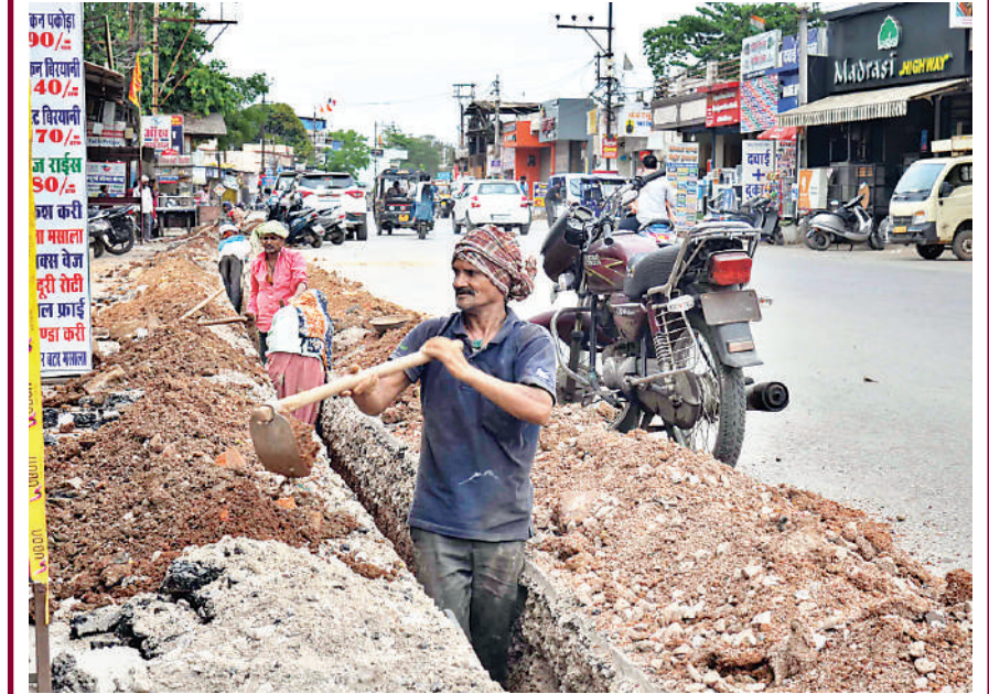
The digging of roads in different parts of capital city is common site for laying of new pipeline and other such works of RMC.
