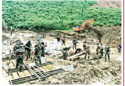
Engineers of Indian Army assist Railway repair teams to reach damaged railway lines for restoration of rail connectivity in North-Eastern states. Extensive cartwork is also done to make a causeway for River Mahur, in Assam's flooded Dimalasas district.
