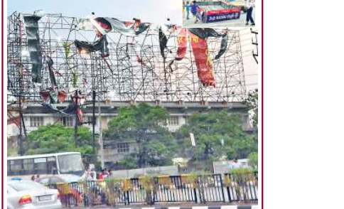
The flexes in the hearings were blown off and cover of round-about of Traffic Police Box was also blown. On Monday evening when strong winds and light showers lashed capital city here
