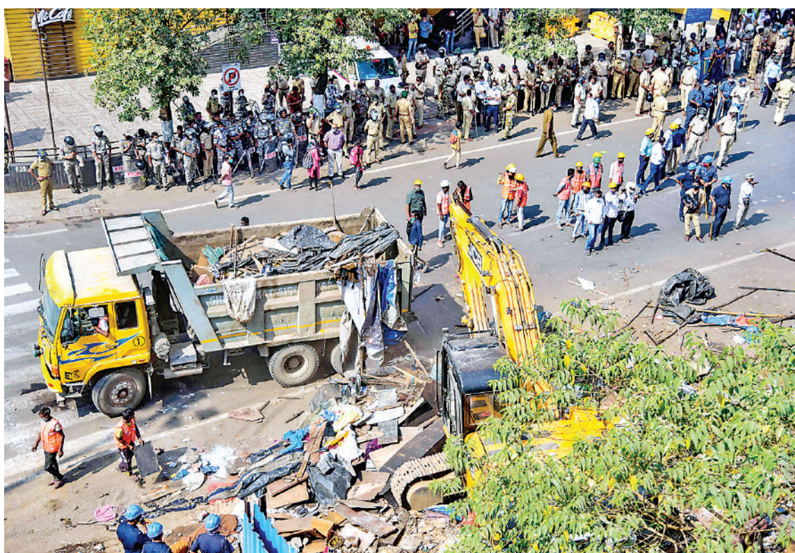
Heavy Police bandobast as NMMC and CIDCO jointly conducts a demolition drive of illegal slums near Kopar Khairane railway station, in Navi Mumbai, Thursday.
