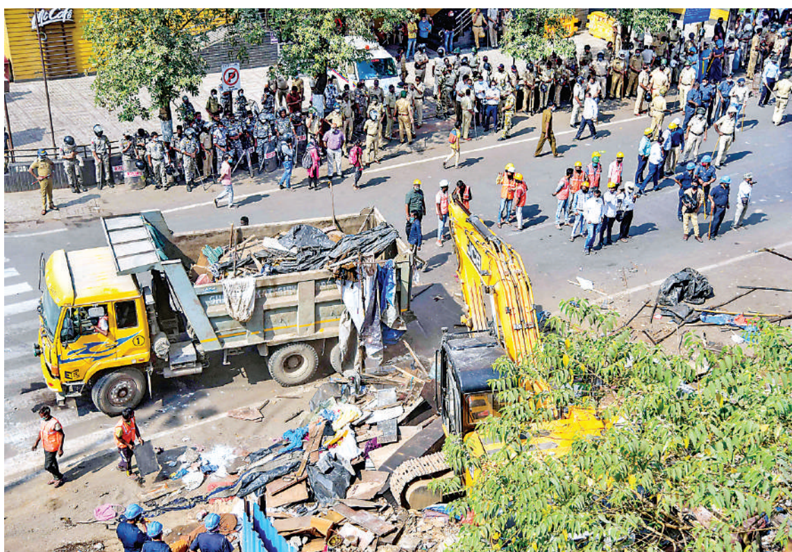
Heavy Police bandobast as NMMC and CIDCO jointly conducts a demolition drive of illegal slums near Kopar Khairane railway station, in Navi Mumbai, Thursday.
