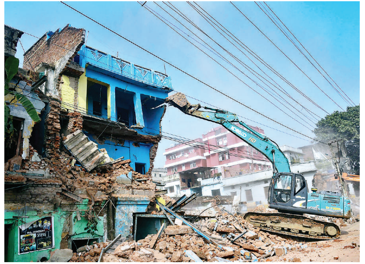
Workers operate an excavator to demolish a building during an anti-encroachment drive at Mithapur area, in Patna, Sunday.
