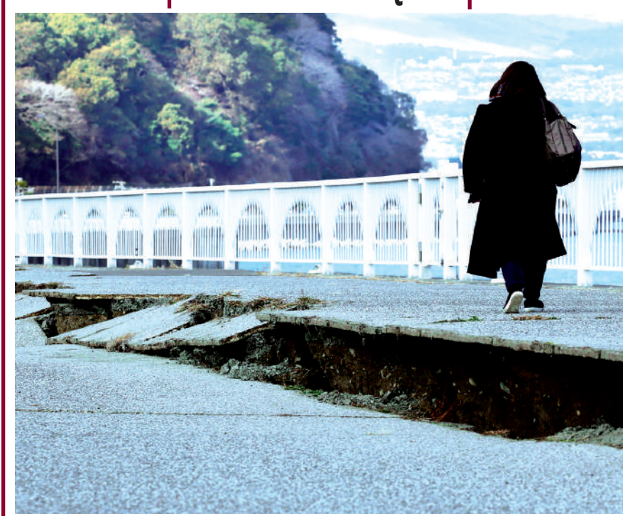
A woman walks along a cracked road in Oita after a 6.4-magnitude earthquake struck off the Pacific coast in southwestern Japan, on Saturday.
